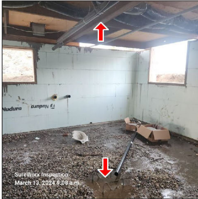
1.2 Item 1 (Picture) Missing post
