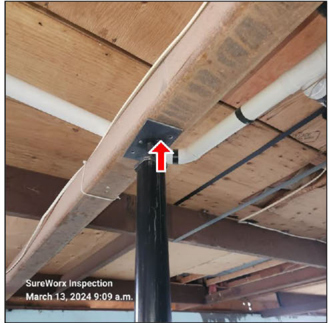
1.2 Item 2 (Picture) Not secured to beam.
