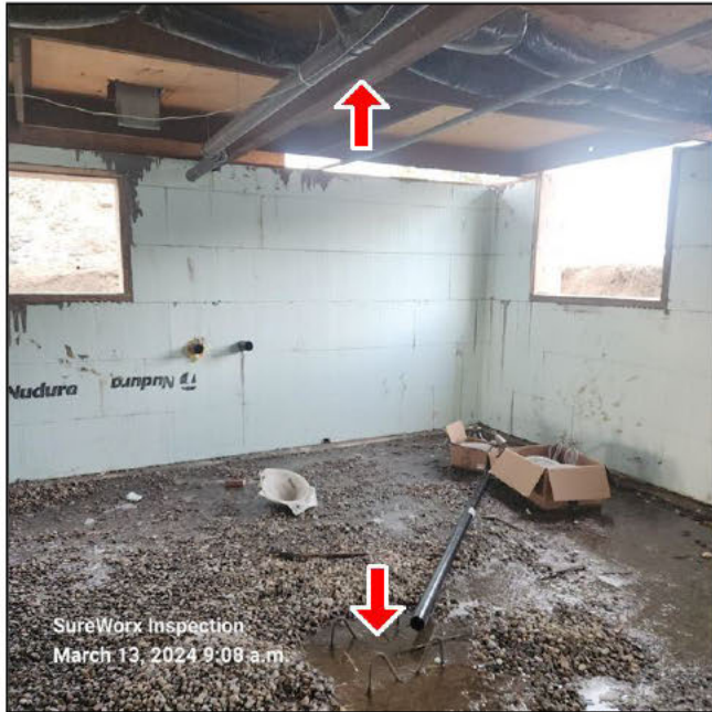
1.2 Item 1 (Picture) Missing post
